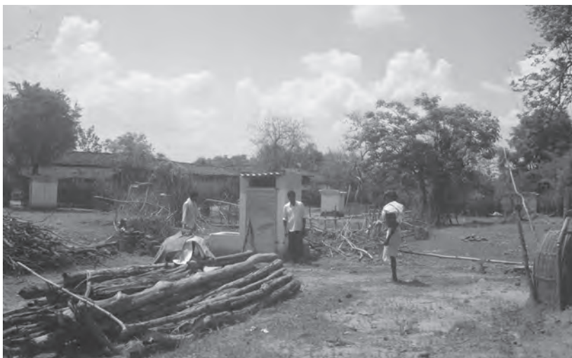
Image D9.1 Building a toilet in India in a rural setting (Sulakshana Nandi)
